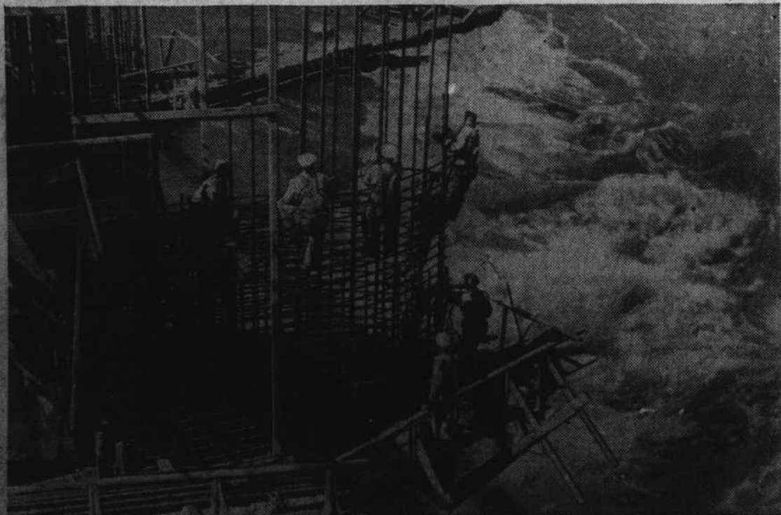
Army engineers are speeding the construction of the $32,400,000 Bonneville dam in the state of Washington. This interesting picture in which sky, water and steel meet shows workers erecting piers that will span the Bonneville river. This PWA project is a huge power, navigation and flood-control undertaking.
