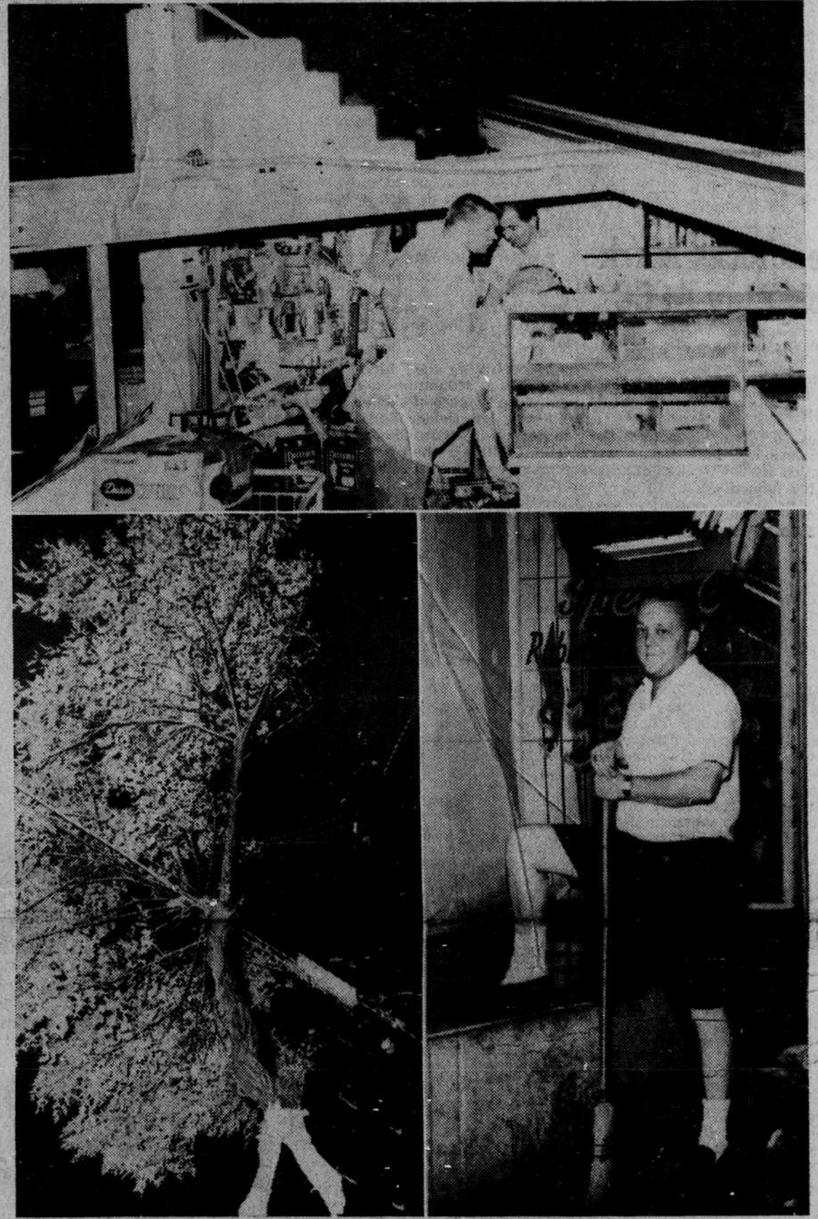
OPEN AIR MARKET - Pictured at top is the remainder of Charles Blalock's Supermarket on Shelby Road after a wind storm Sunday night in which the building collapsed. Lower left is one of several limbs and/or trees blown into electric lines. Lower right, Bob Ramsey, manager of City Paint Store, mops up damage done to his store window during the high winds which reached tornadoic force. Damage done by the storm has been speculated at near a half-million dollars. (Herald Photos by Claire Gilstad)
