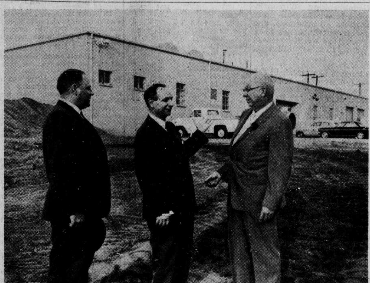
MANUFACTURER IN MAJOR EXPANSION - Ground was broken recently for a 33,000 square foot addition to Duplex-Shannon, Ltd., a new firm resulting from the merger of Kings Mountain's Shannon, Ltd., and New York's Duplex International. Pictured at the construction site with the
