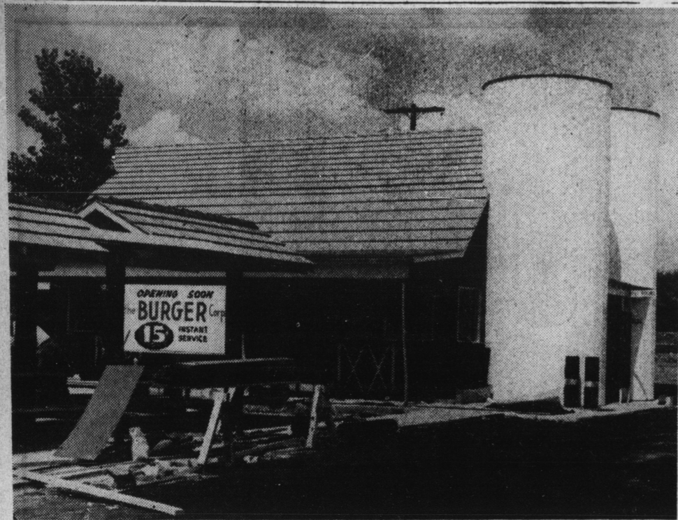
OPENING THURSDAY — Workmen were busy this week putting the finishing touches on the Burger Barn, located on York road, a new short order firm, which will open Thursday morning.
