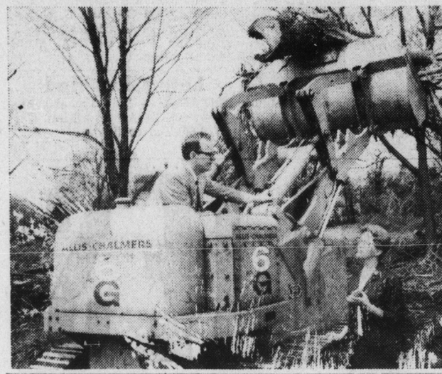
GRADING UNDERWAY — Fifty percent of the grading has been completed at site of the new home of Kings Mountain Savings & Loan Association at the corner of S. Casler and Mountain streets. Ground was broken last Wednesday, and despite bad weather several days this week, a clay and cinder foundation has been laid. Joe R. Smith, executive of the firm, sits in the driver's seat of the equipment being used to do the grading work. Observing the proceedings is Mrs. Philip Baker, an officer of the association.
