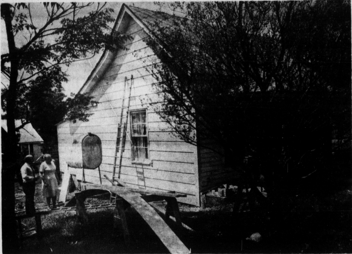
REHAB UNDERWAY —Reg Alexander of the KM Housing Rehabilitation Program and Mary Dover look over the rehab work underway at her Bennett Dr. home. The home is about 100 years old. Mrs. Dover has
