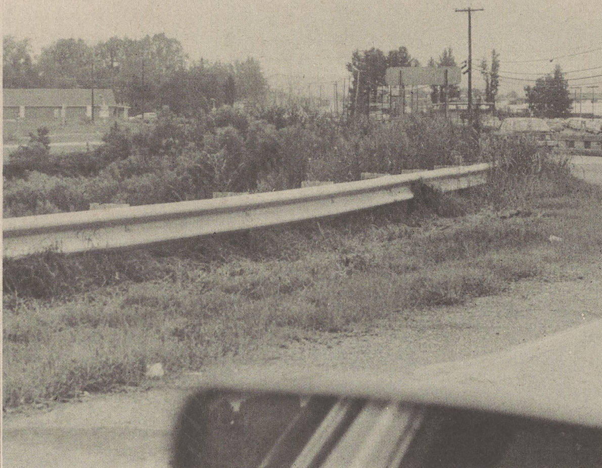
DANGEROUS INTERSECTION —Motorists coming onto the exit ramp at Interstate 85-Highway 161 and attempting to make a left turn toward Kings Mountain have difficulty seeing southbound traffic on Highway 161 because of high weeds, grass and other growth along the bridge.
