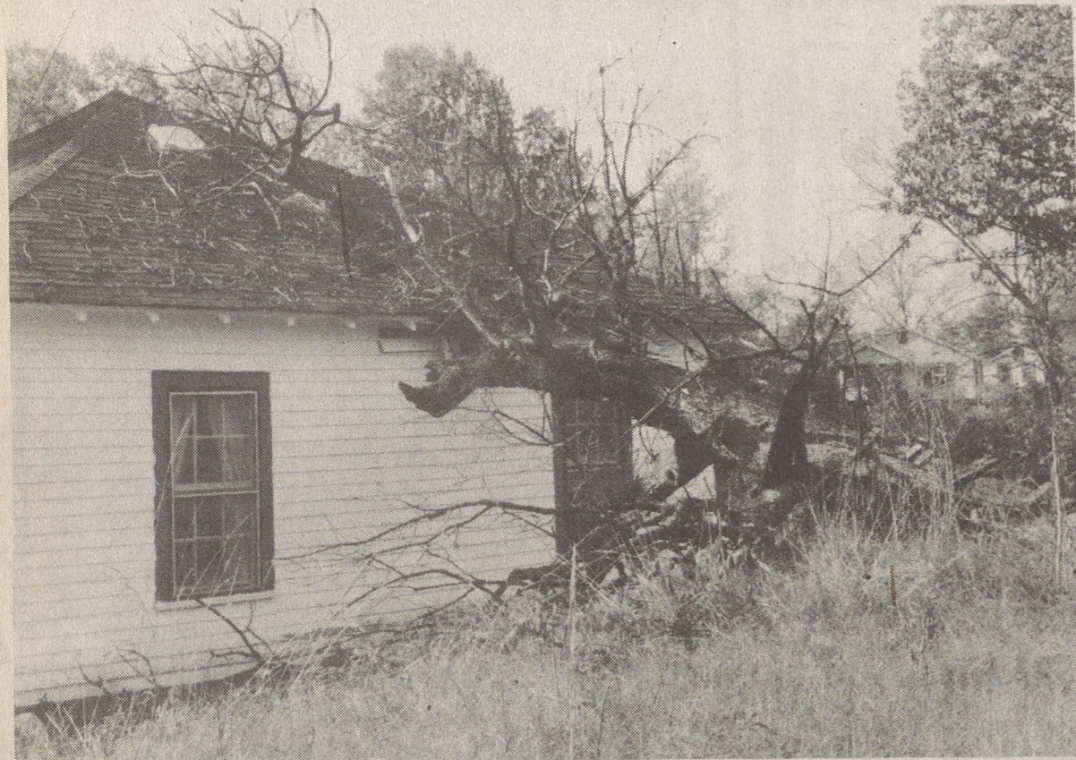
HOUSE DAMAGED WHEN TREE FALLS —The home of Mr. and Mrs. Charlie Taylor on Ellison Drive was damaged Friday morning when a tree on a neighbor's lot fell. Mrs. Taylor, inside the house at the time, said she heard a loud noise and went outside and saw the large tree had fallen on the top of her house. The Taylors rent from Eugene Roberts. The tree fell from the property of Loretta Lee Ware, formerly of 205 Fairview Street. After her house burned, the Ware property was condemned by the city but efforts to contact the owner have been unsuccessful. City codes officers in May 1985 ordered the owner to clean up the property. The Taylor house is insured.
