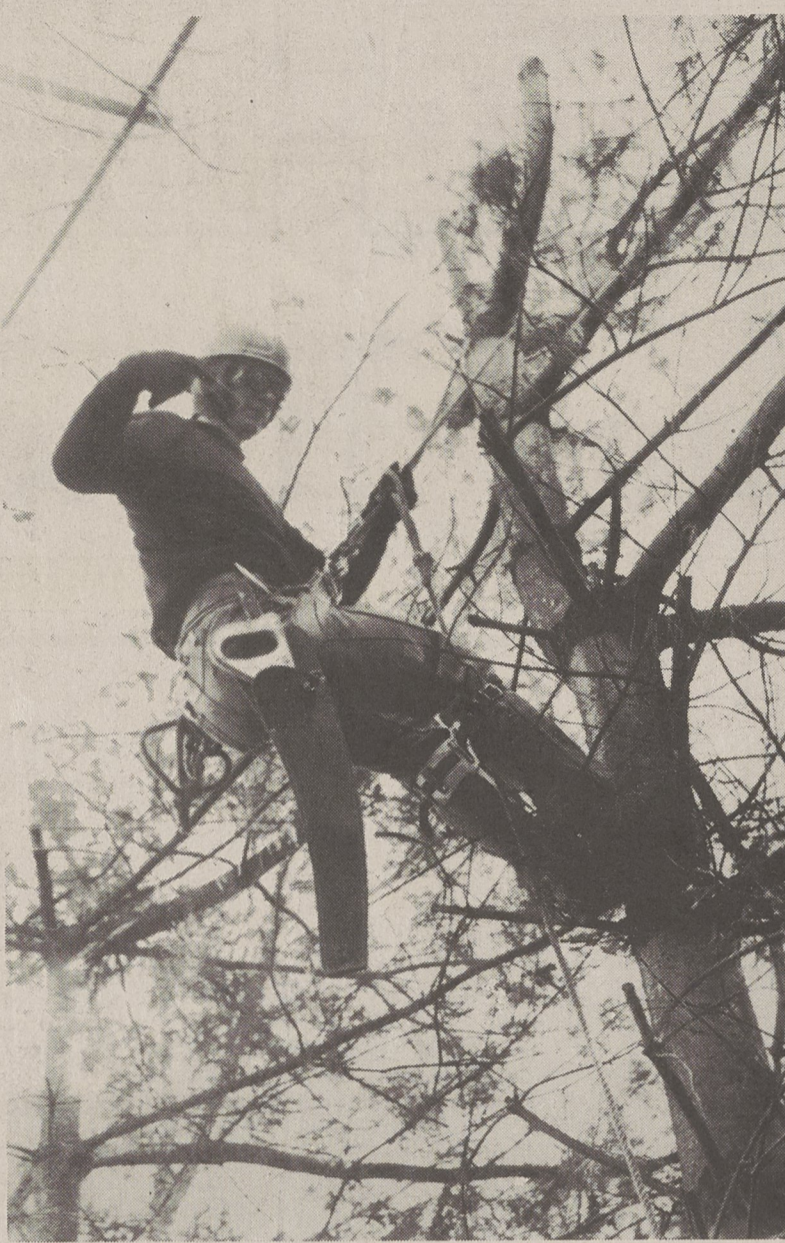
ELECTRICAL WIRES - Crew began cutting out limbs from the worst areas first.
