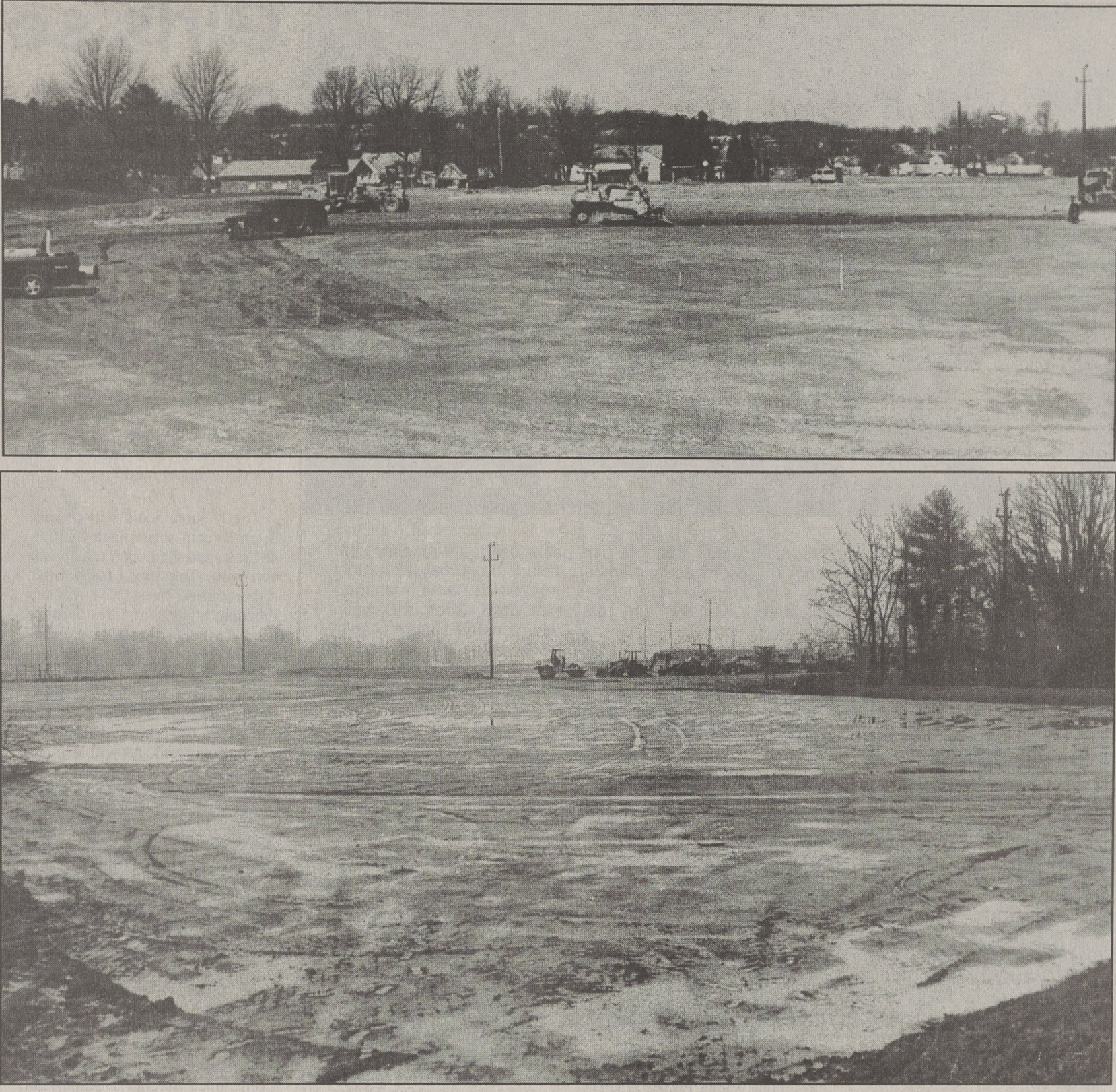
WORKING ON BASEBALL FIELDS - Employees of Champion Contracting (top photo) are hard at work fine-grading the new baseball fields at Deal Street Park, but one good day of work is usually followed by a day of rain which turns the fields into a huge mud hole (bottom photo).
