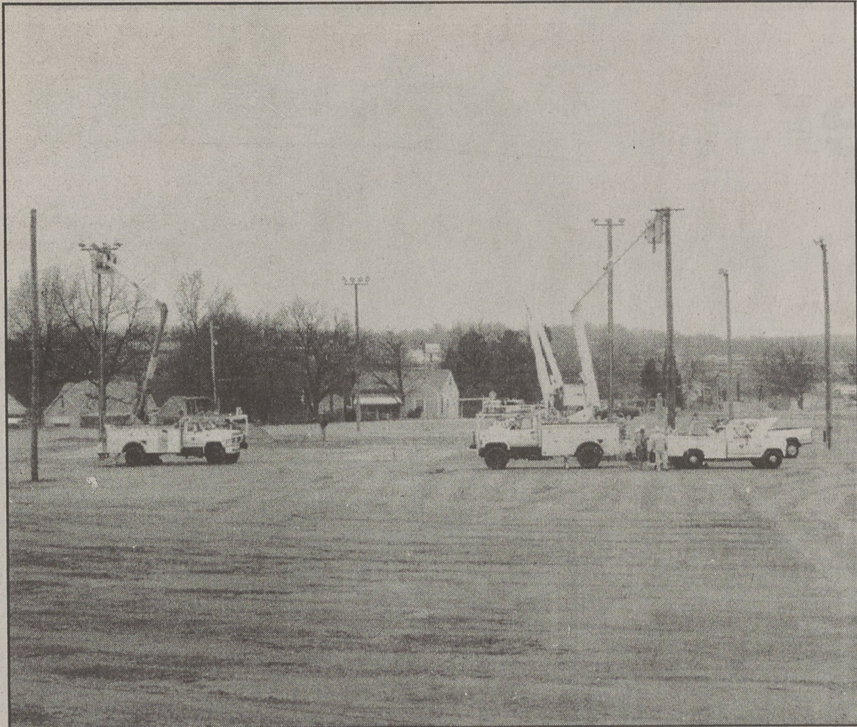
LIGHTS GOING UP - Kings Mountain electrical crews put up lights and poles on the new Deal Street baseball/softball complex Monday. The fine-grading and some of the seeding of grass is completed and the city hopes to have the fields ready for the start of Dixie Youth League play in the spring.
