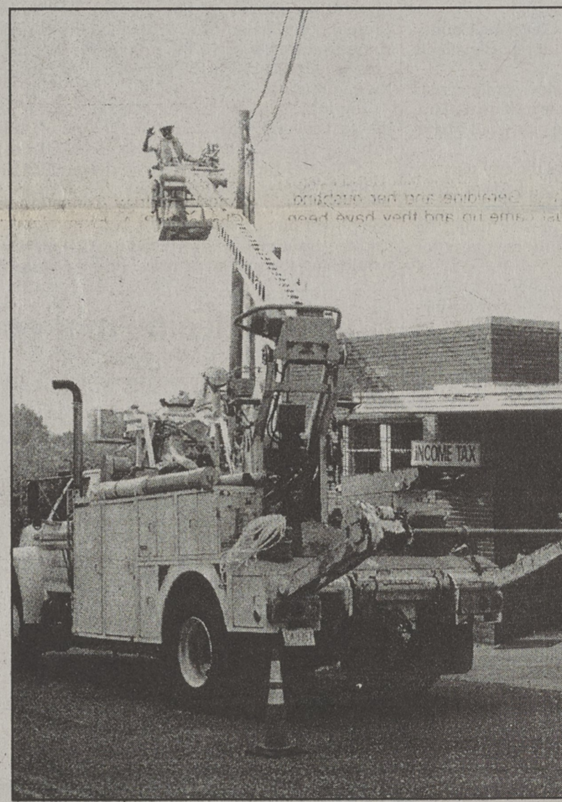
GETTING READY - Larry Davis of Bell South works from a bucket truck to hook up communication lines which will serve the Kings Mountain Police Department when it moves to the old Herald building on S. Piedmont Avenue.
