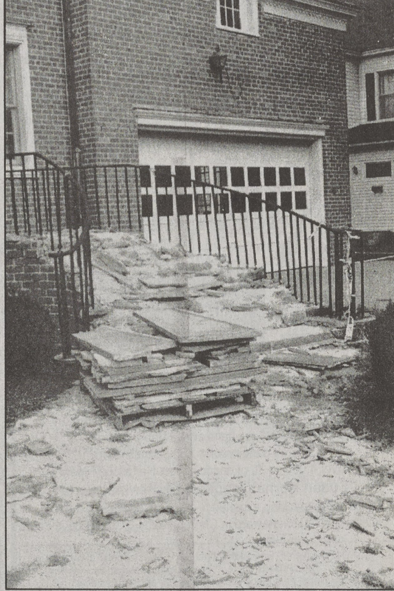
CITY HALL DISAPPEARING - The old Kings Mountain City Hall/Law Enforcement Center is quickly disappearing. City firemen are removing and salvaging the old concrete steps in front of the building to be used at the fire museum. The firemen also last week salvaged the cupola and police communications tower to be used in the future at either the fire museum or a new fire station. Soon the building will be demolished and the lot cleared to make way for a new $1.6 million law enforcement center.
