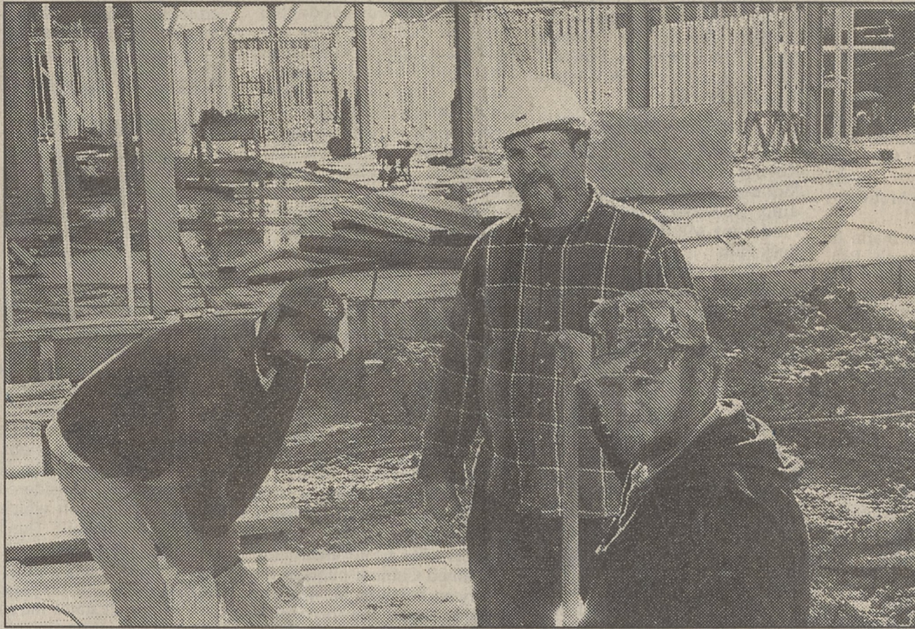
Michael Henderson, Milo and Ronnie Hawks are hard at work laying pipe at the new Kings Mountain Police Station. The city hopes to get the building "in the dry" before the bad winter weather hits and have it ready for occupancy later in 1999.
