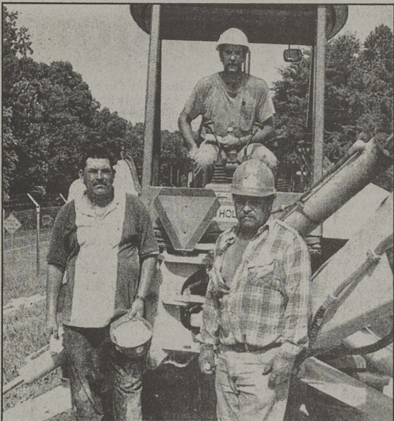
Backhoe operator Scott Sullivan and his helpers Juan Saldina (left) and Mario Calvillo were doing their dusty duty recently at Moss Lake with crews hooking up the new Kings Mountain water main. Sullivan is from Wingate and his men are from Monroe.
