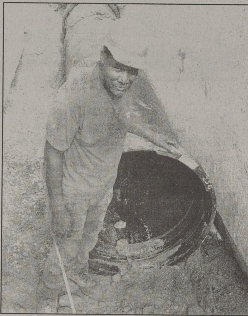
Jerry White of Crowder Construction gets ready to clean out the new water main that will go to Kings Mountain from Moss Lake.
