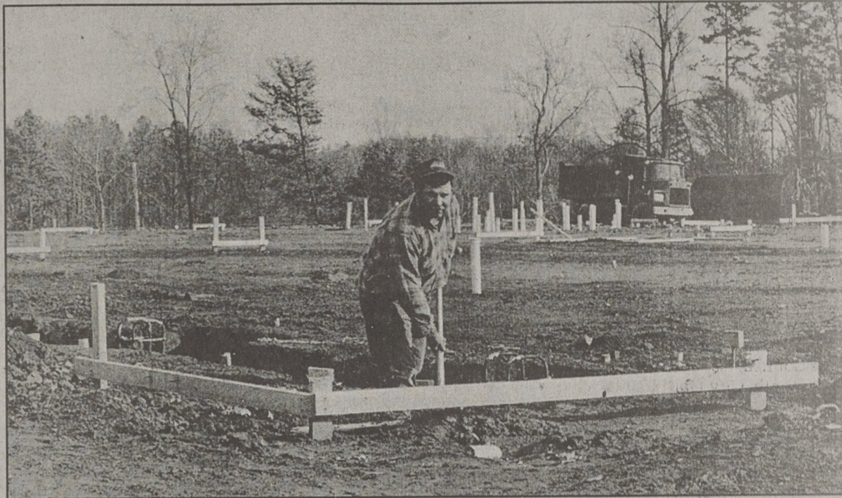
ALAN HODGE/THE HERALD On the job recently at the new Kings Mountain Senior Center, worker Millious Holland was smoothing out some foundation trenches. An evening shower had made for a rather muddy day.
