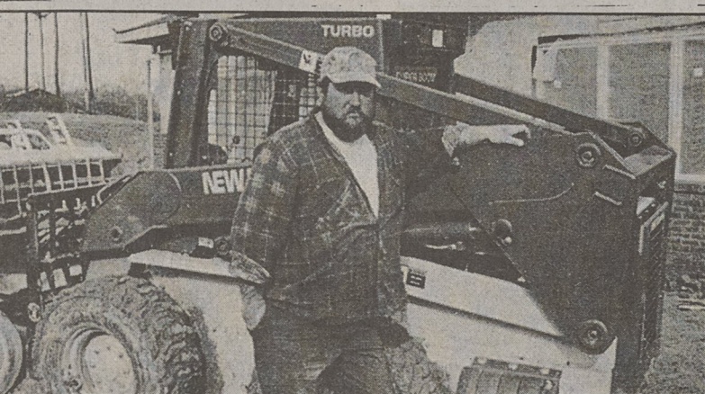
ALAN HODGE/THE HERALD Worker Mark Hunt was getting ready to fire up this piece of machinery at the site of the new Kings Mountain Woman's Center. Hunt said the recent good weather had speeded up the job.
