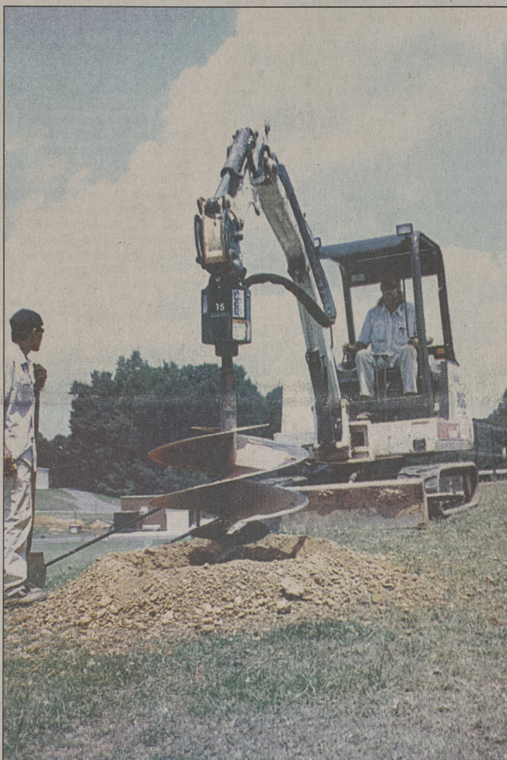
GARY STEWART / THE HERALD David Cooper, left, and Robbie Chapman of Fountain Electric of Spindale drill 15-foot deep hole at John Gamble Stadium, where new lights are being installed this week. The light project, which is costing $100,000, includes underground wiring and will be completed in time for the high school football season which begins August 18 with the Cleveland County Jamboree.
