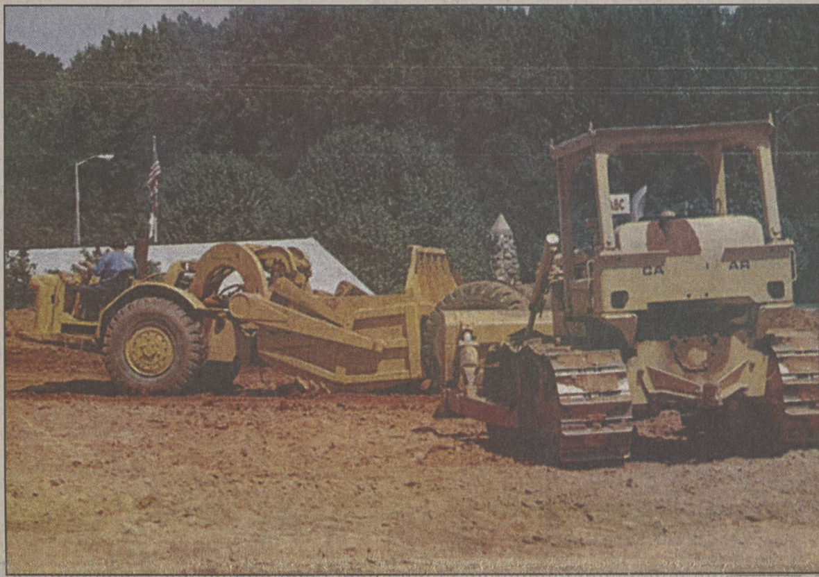
BEN LEDBETTER/THE HERALD Preparations for the September playground build dates move forward as workers perform grading work recently at the playground site on Cleveland Ave.
