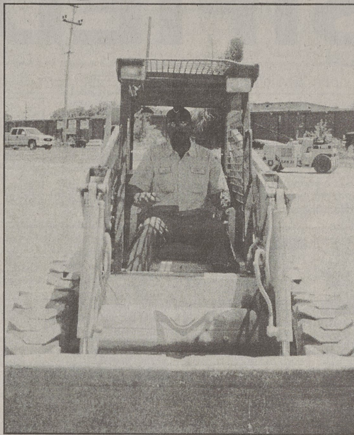
BEN LEDBETTER / THE HERALD Cearcil Reid prepares to operate the skid steerer at the site of the new family life center at East Gold Street Wesleyan Church.
