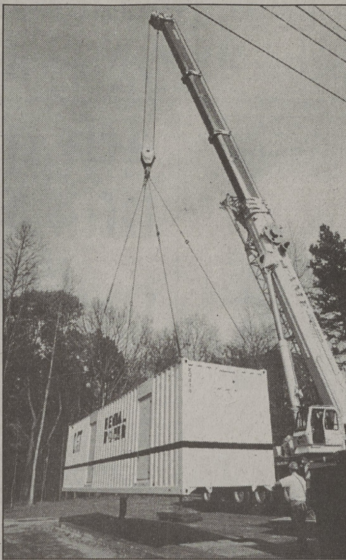
ELLIS NOELL / HERALD A huge crane lifts one of the electric peak shaving generators into place Thursday at the electrical substation off York Road in Kings Mountain.
