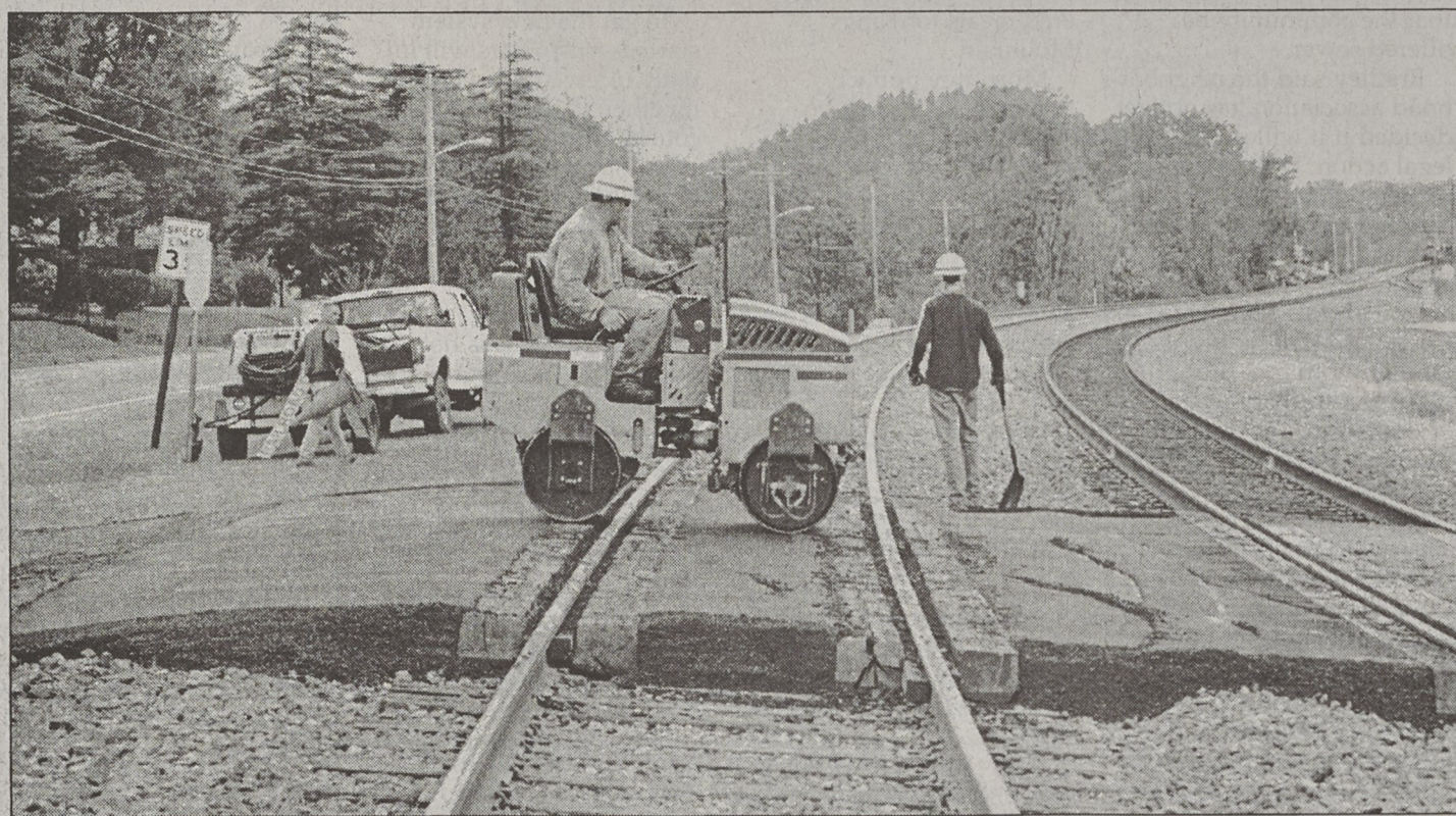
GARY STEWART / HERALD Southern Railway is doing maintenance work at several crossings in Kings Mountain this week, replacing some cross ties, adding rock and repaving crossings. Above, workers are shown Tuesday repaving the crossing at Parkdale Mill. In the background is the Hawthorne Street crossing which was also improved later Tuesday.
