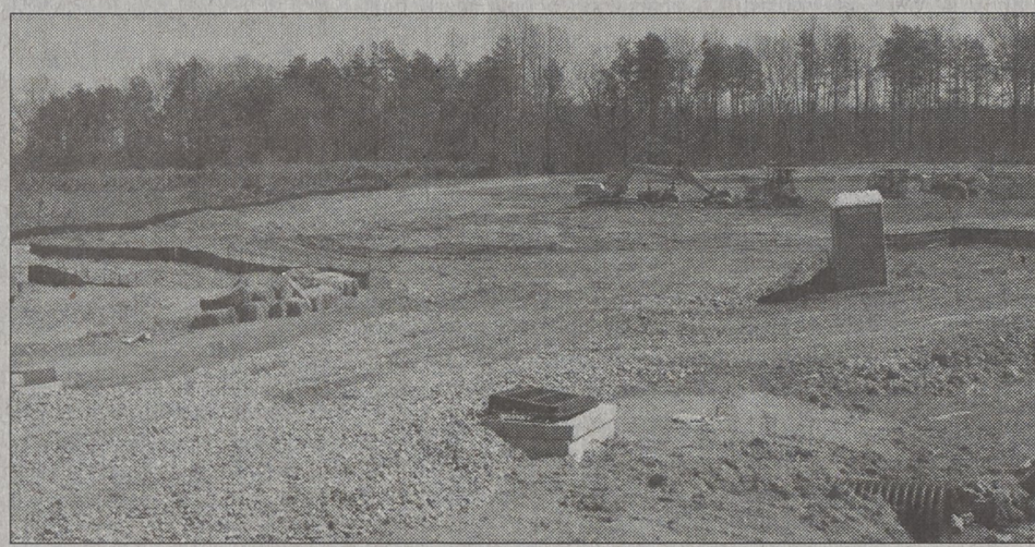
Photo by EMILY WEAVER Construction is underway at the future site of the Kings Mountain Hospice house on Kings Mountain Boulevard.
