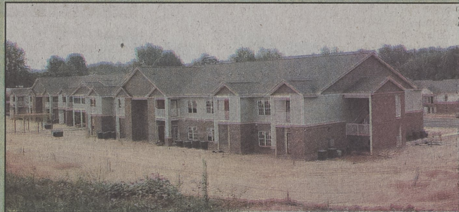
photos by EMILY WEAVER The 84-unit E. Gold Street apartment complex is springing up nicely. Construction workers for Pendegraph Company of Greensboro have been working at the site and have made a lot of progress since March when foundations were being poured and walls were just starting to go up. As seen in the photograph taken Tuesday morning, several units are already up and finished (from outside appearances) and parking lots are being formed. The new housing, expected to be completed this year, will provide 38 units for senior citizens.
