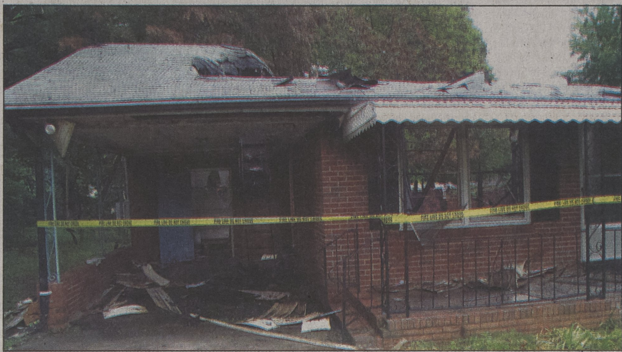
Arson is suspected in a mysterious fire that destroyed a vacant home on Silver Street on May 13. Officials suspect gasoline may have been used. The case is still under investigation. KM-Fire Chief Frank Burns said the house was fully engulfed by flames when firemen arrived at the scene. The State Bureau of Investigation was called in to help with the investigation.
