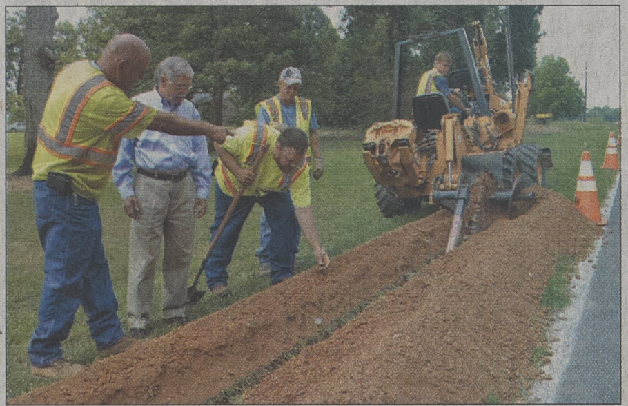
photo by ELLIS NOELL The City of Kings Mountain is expanding its natural gas line 3-5 miles every year to offer gas service to citizens who want to hook on. Here, city workers work on a new line on Brooks Road after completing infrastructure on Battleground and Canterbury Roads. City officials are looking at extending a loop on Rollingbrook Road. From left Daryl Philbeck pointing to the new line, Mayor Rick Murphey, Chase Gibson, Terry Cain, and Nathan Deal.
