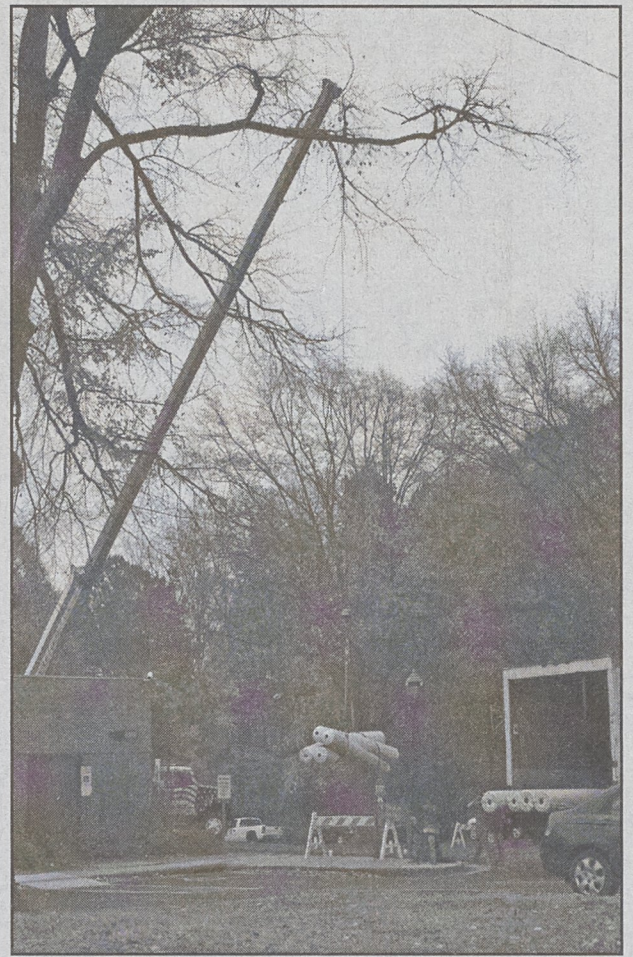
Workers load roofing material onto City Hall last Friday. After years of expensive leaks, the city is replacing the building's roof in a job that could take a month if bad weather interferes with the project.
