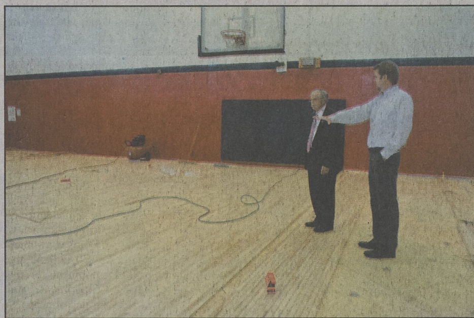
Mayor Rick Murphrey, left, and Kings Mountain Family YMCA Executive Kevin Osborne inspect the construction of the new gymnasium floor expected to be ready for the November 15 opening season of basketball at the Y. The renovation, which includes new bleachers, will mean two basketball/volleyball teams can play at the same time in the gymnasium allowing more participation at the facility.
