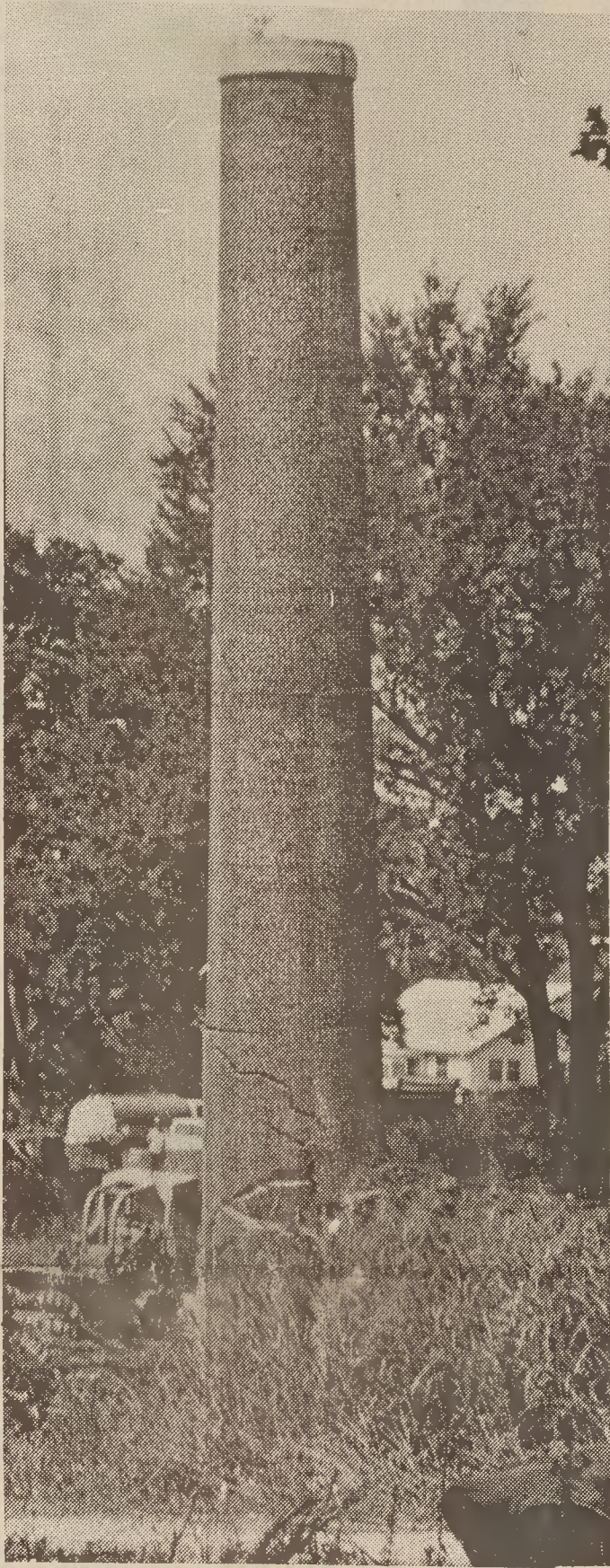
GOING DOWN, PLEASE — The 94-foot high Bonnie Mill smokestack fell to rubble Tuesday morning during demolition of the property by Bradley-Jenkins Enterprises employees. The mill is one of 30 structures coming down under a $53,000 demolition contract from the city's redevelopment commission.
