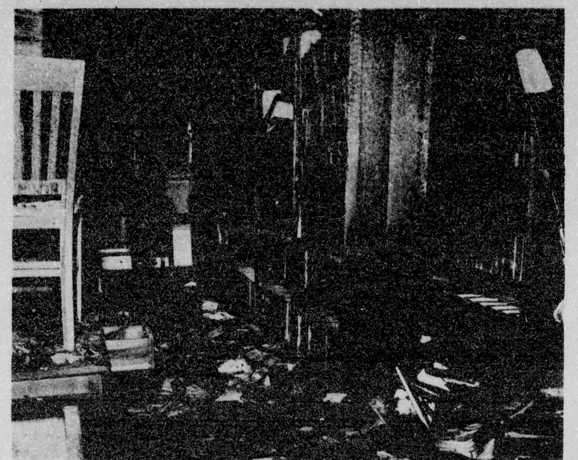
NCCU LAW SCHOOL FIRE DAMAGE - Damage figures were not complete Monday as cleaning up of the debris left by the disastrous fire at North Carolina Central University's law school began. The fire, early Friday morning, destroyed as estimated $500,000 worth of law books, including irreplaceable volumes dating from the 18th century. A former NCCU law student was held by police in connection with the blaze.
