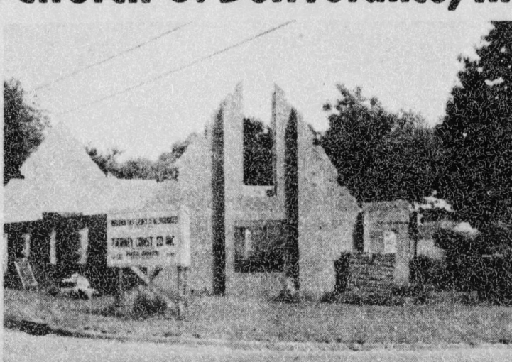
THE WESLEYAN FIRST CHURCH OF DELIVERANCE, above, is nearing completion. Funds are being sought at this time for its completion. Raleigh's well-known Sister Mable Gary is the pastor.
