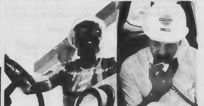
BULLDOZER DRIVER, TRAINING DIRECTOR — Mrs. Edith Finch of Raleigh, is shown at the wheel of a bulldozer, while Bill Parker of Garner, right, director of training for C.C. Manguam Construction Co., Raleigh, looks over a work sheet. Many women, both black and white, are now engaged in the construction trades. (Staff Photos By Joyce A. Bass)
