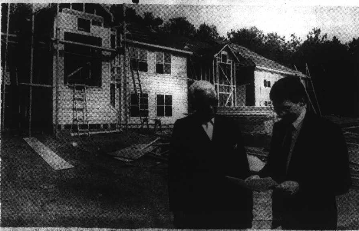
AFFORDABLE HOUSING —Gregory Warren, executive director of Downtown Housing Improvement Corp. (DHIC) and John "Top" Green, a member of the board of directors, review plans and discuss progress of the Jeffries Ridge
