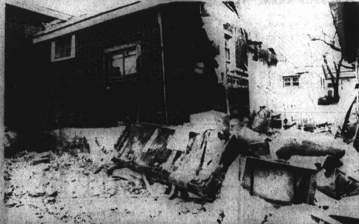
HOUSING DECAY—Just blocks from downtown Raleigh, this Cabarrus Street home is an example of the extreme
