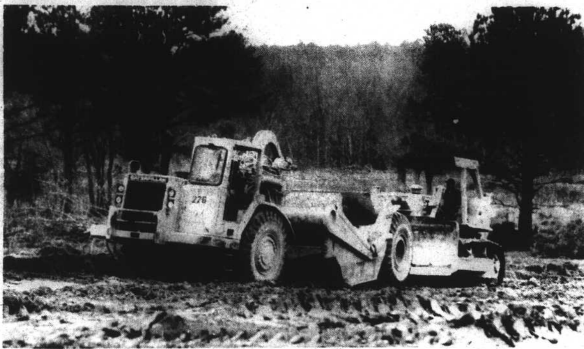
THE CLEARING —Clearing has begun at Walnut Creek Amphitheater, a $13.5 million open-air performing arts center featuring both reserved seats and festival lawn-seating. The facility will be centrally located in Raleigh's new Walnut Creek Park, just southeast of the Beltline near I-40 at the intersection of Rock Quarry Road and Sunnybrook Road. Opening scheduled for July, 1991.
