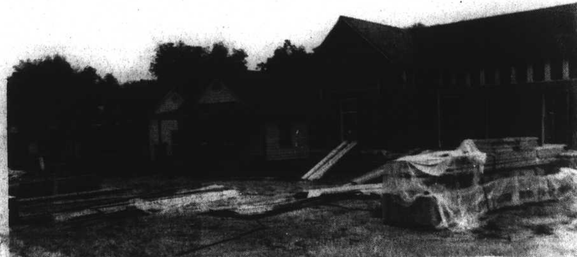
A NEW BEGINNING—Shown above are several new homes that have been constructed over the past weeks as part of the City's Enhancement program to develop part of Chavis Way. The United States Congress has passed a new Housing Program and it includes an authorization for funds to cities in a Block Grant Program known as "Home".
