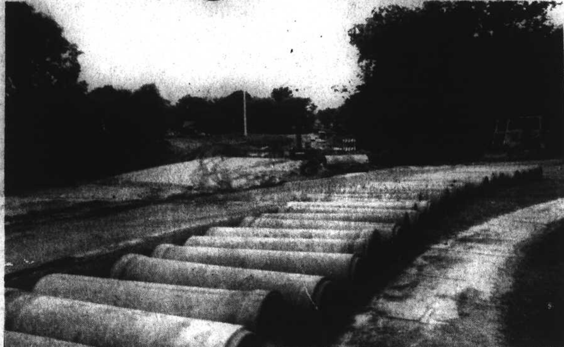
M. L. KING EXTENSION UNDERWAY—The new extension is taking place from Rock Quarry Road top S. Blount Street. Boundary and Smithfield Streets along with a segment of Garner Road will be renamed M. L. King Boulevard.
