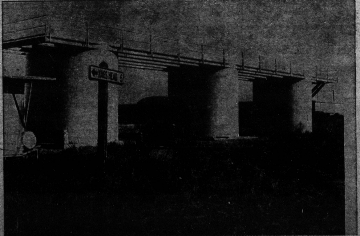
WORK IS WELL UNDERWAY on the missile tracking station shown above which is located off the Oregon Inlet road five miles south of Nags Head. Construction began on the site Nov. 11 and is not expected to be complete for several months. The three towers in the photo are 15 feet tall and 16 feet in diameter and are constructed of steel sheets supported by beams. The galvanized catwalks above the towers will be used to support cameras, radar antennas and other equipment. The drum-like towers are unique and were necessitated by the shifting sand conditions on the coast.
