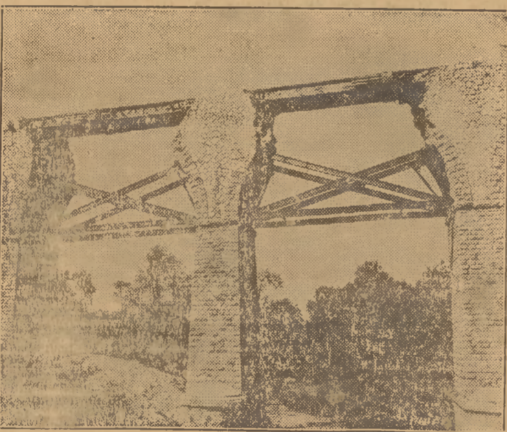
Four days later Pont de l'Arc was repaired and trains were in operation carrying stores and munitions to advancing American troops.
